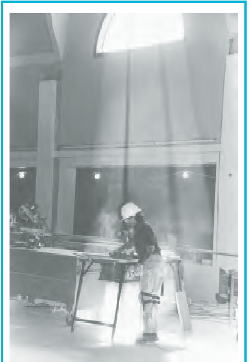
BLESSED WORK —A workman in the sanctuary of the nearly completed new Holy Apostles Church, Chinden and Meridian Road, Meridian, is bathed in sunlight, which is coming through a high southern window. The parish expects to use the church building for Easter services the weekend of April 15. (ICR photo by Colette Cowman)
