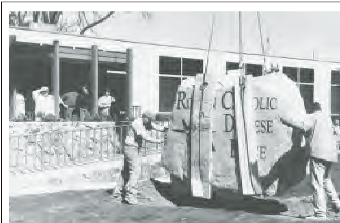
'A PIECE OF THE ROCK' —Workmen install a nine and a half ton rock—a ton and half heavier than the average African elephant—May 4 in front of the Diocesan Pastoral Center in Boise while staff members watch. The lighted rock, some of which was donated by John and Catherine Englund
