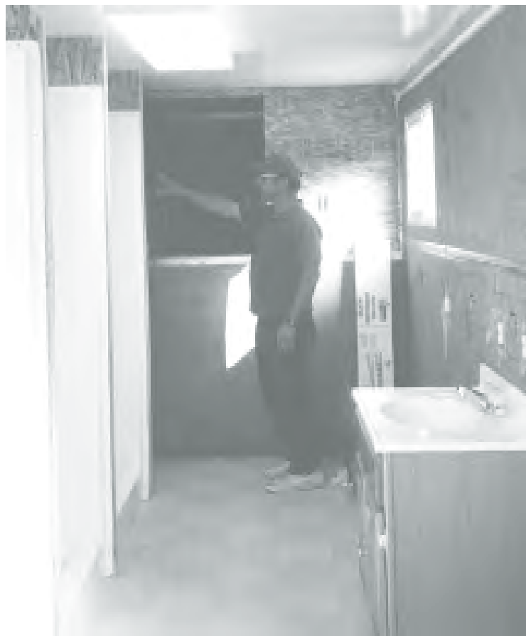
CURSILLO SHOWER TRAILER — Marvin Mackay checks out one of the shower stalls in the trailer volunteers from the Cursillo movement are remodeling so that participants in Cursillos and retreats will have adequate shower space. (Photo by Karma Fitzgerald)
